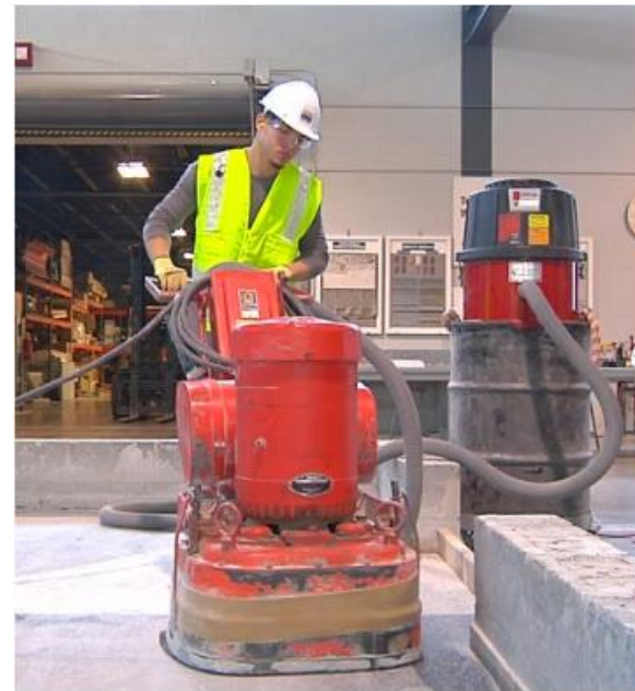
Worker milling granite floor indoors with milling machine and dust collection system (background).
