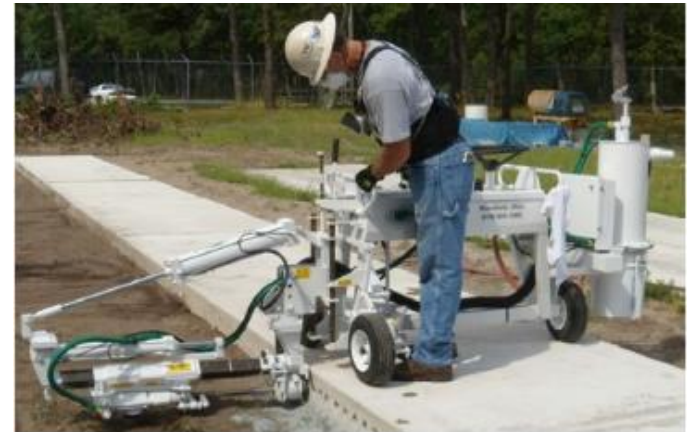
Worker drilling horizontal holes in concrete slab with a dowel drilling rig. The shroud surrounds the drill steel where it enters the concrete and the dust collector is the canister on the right. Worker is wearing respiratory protection.
