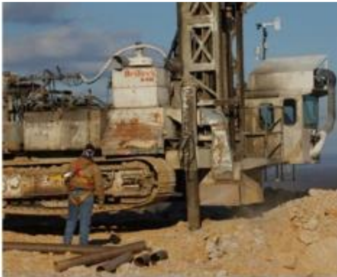
Vehicle-mounted drilling rig using water on the drill bit. The enclosed operator's cab is on the right.
